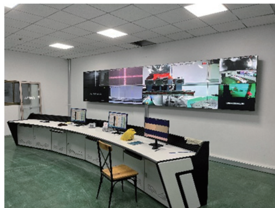
Fig. 2 (color online) The Control room.
