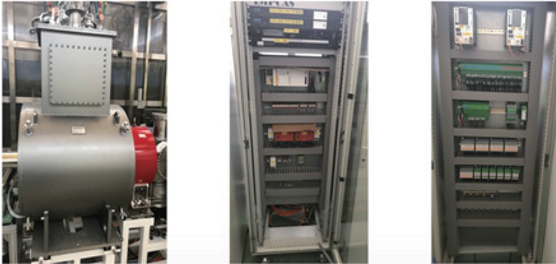
Fig. 1 (color online) HECR and its control system at IMP.
