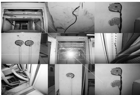
Fig. 1 T/H module installation places.
