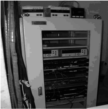
Fig. 1 Picture of controllers modules.
